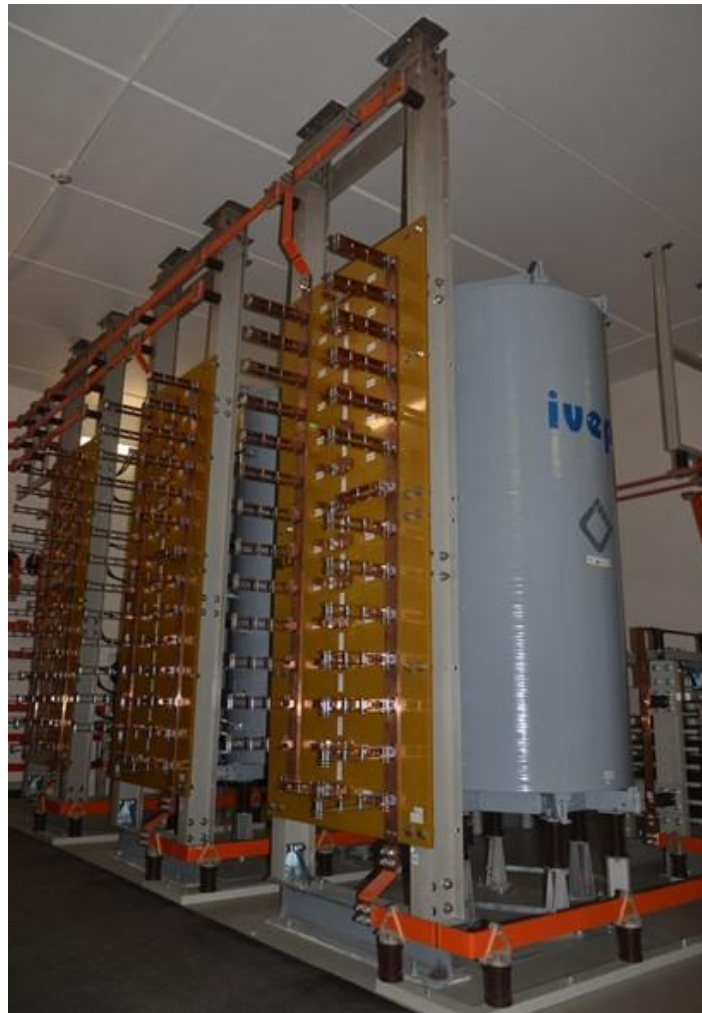
Fig. 2: High voltage part of the High Current Laboratory
