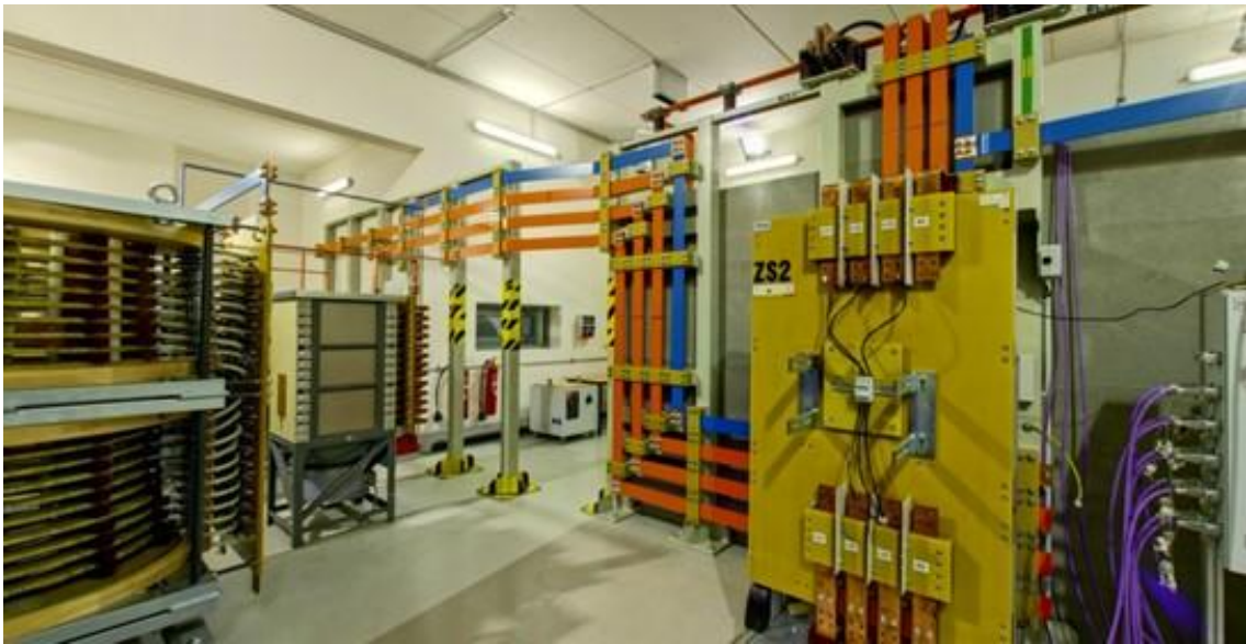
Fig.1: LV part and testing bench of the High Current Laboratory
