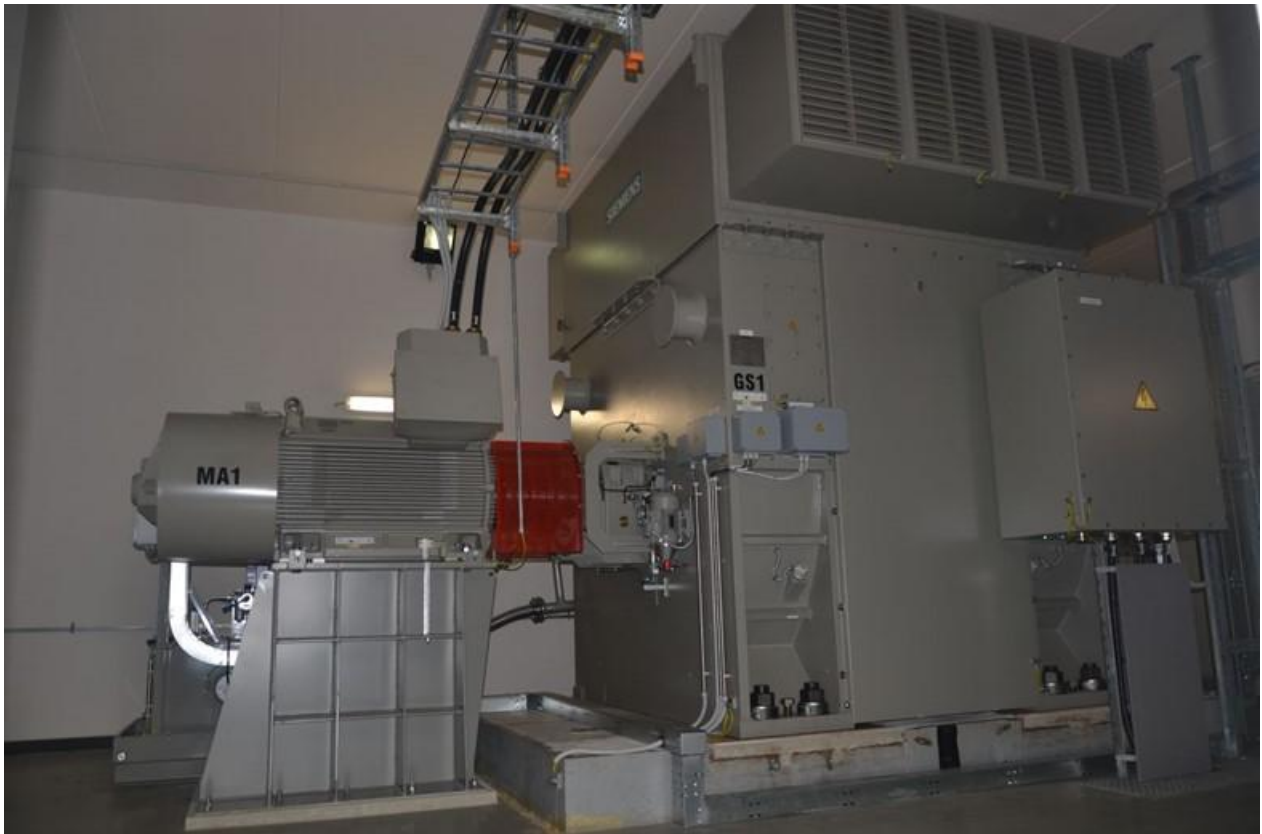
Fig.3: Generator of the High Current Laboratory
